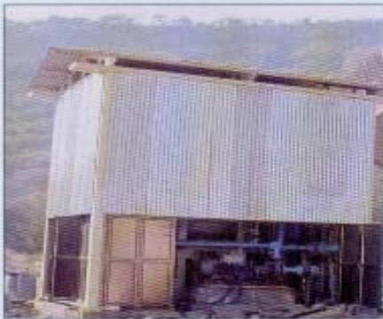
Low Temperature Evaporation Plant at CIRUS
