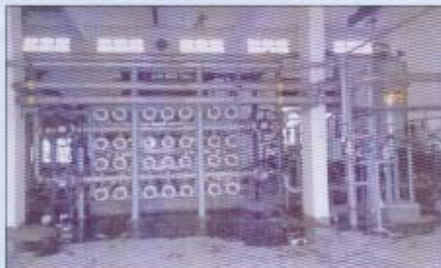
Sea Water Reverse Osmosis (SWRO) Plant building and membrane modules
