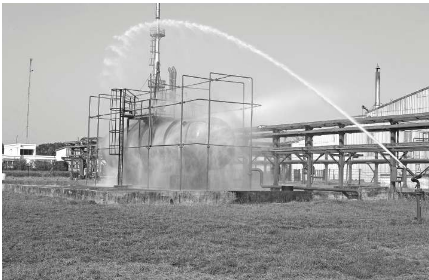
Sprinkler System for Safety
