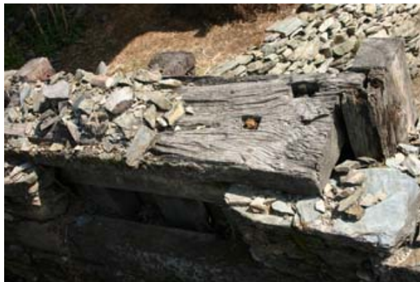
Figure 5. Housed and nailed joints used for fixing the wooden components of the Koti Banal architecture.
